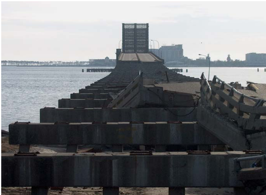
Figure 2. Failure of the US90 bridge crossing Biloxi Bay, Mississippi
