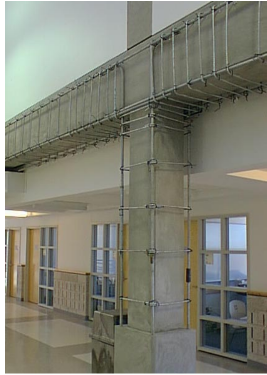
Fig. 2 Exposed re-bar reveals innermost structure of concrete columns and beams
