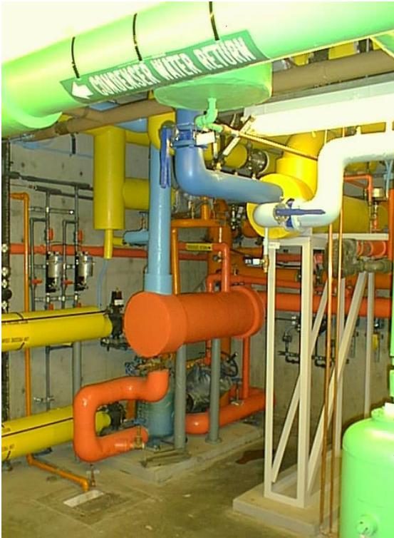
Fig. 1 Mechanical equipment is color coded to identify different systems
