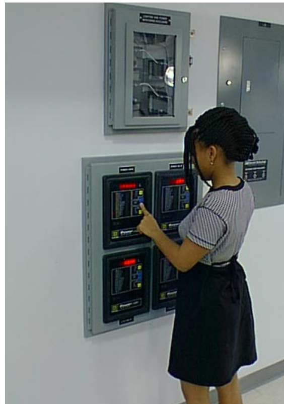
Fig. 4 Square D Power Logic monitors electrical system performance
