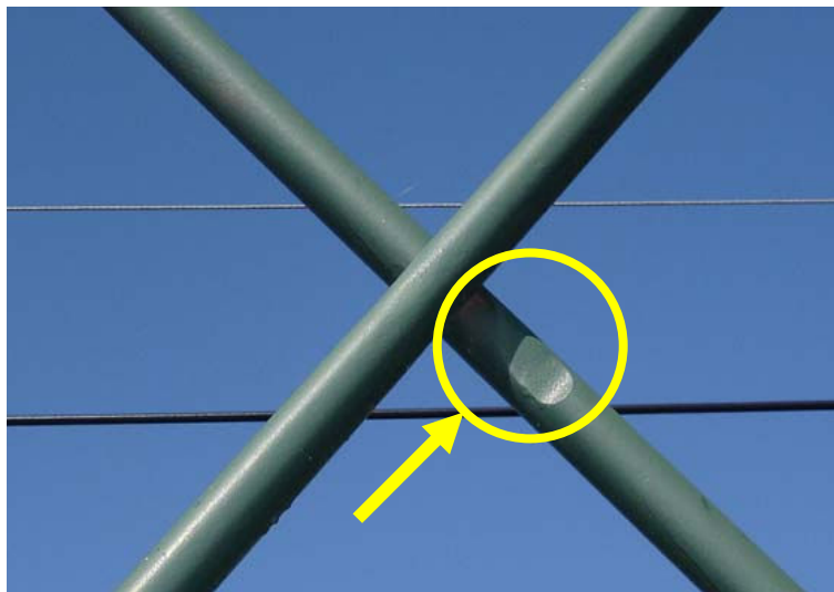
Figure 8. Section Loss on Diagonal Member, Center Bay, West Truss, Span 2.
