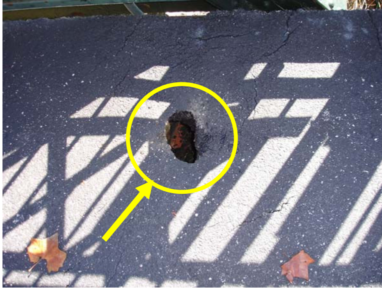
Figure 9. Large Hole in Deck, North End of Span 3 near East Truss.
