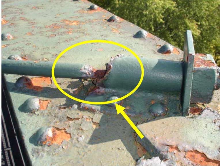
Figure 7. Heavy Section Loss on Upper Lateral Bracing Member, Typical Throughout
