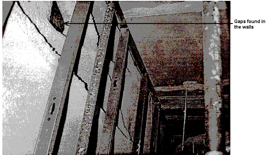
FIG - 4: GAPS FOUND IN THE WALLS
