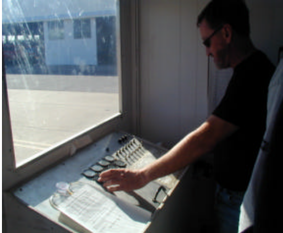
Figure 4 Control panel operation
