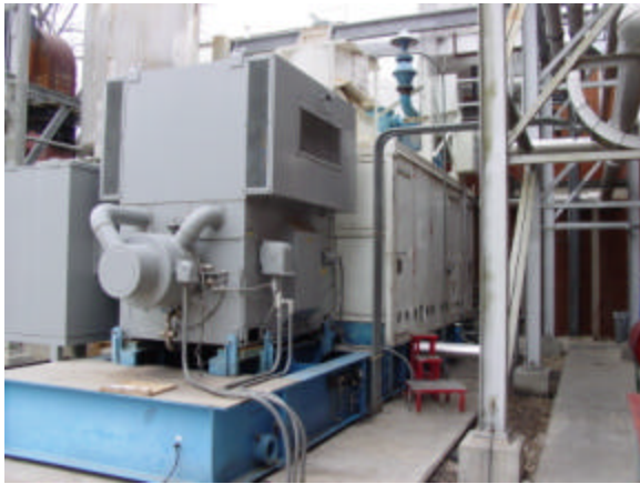
Figure 13 Close-up of the gas turbine and generator housing
