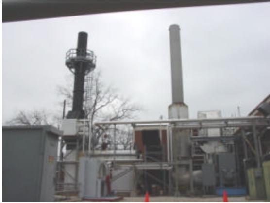
Figure 12 Co-generation power facility
