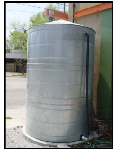
Figure 1. Cistern used for rainwater harvesting in North Carolina (Source: Dwane Jones)
