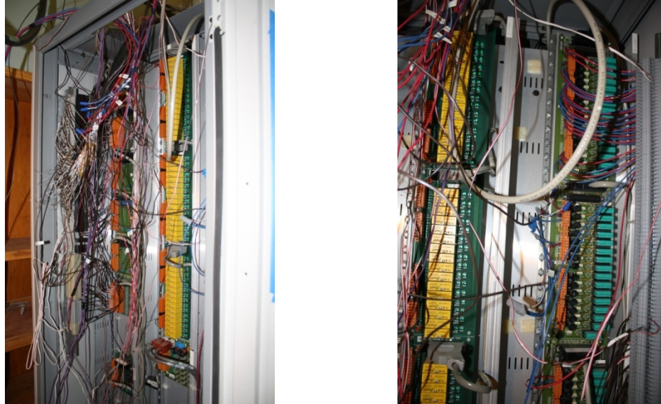
Figure 10 – Wiring of Field Termination Assemblies
