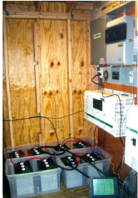
Figure 7. Inside the powerhouse
