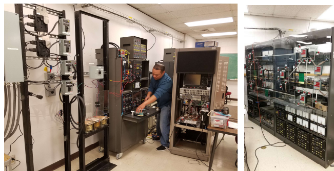
Fig. 3. Power Systems Teaching and Research Laboratory at the New Mexico State University
