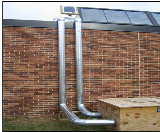
Figure 2 Final Solar Heating System
