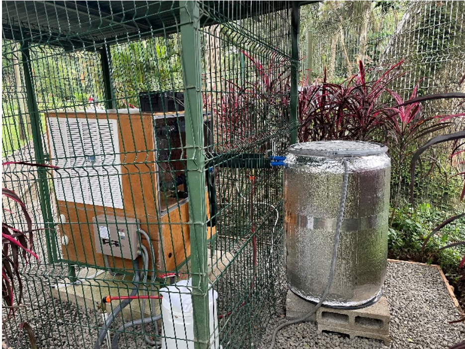
Figure 9: Rear View of the System at the New Location.
