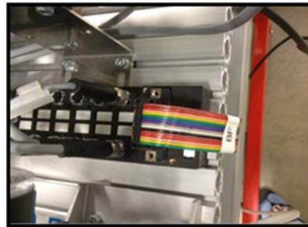
Figure 7. Ribbon cable connections between Easy Port and field devices
