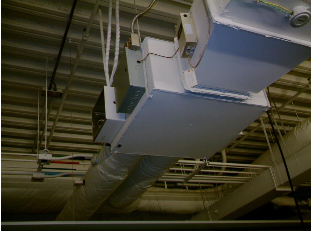
Figure 5.0, VAV Mixing Box suspended from ceiling.
