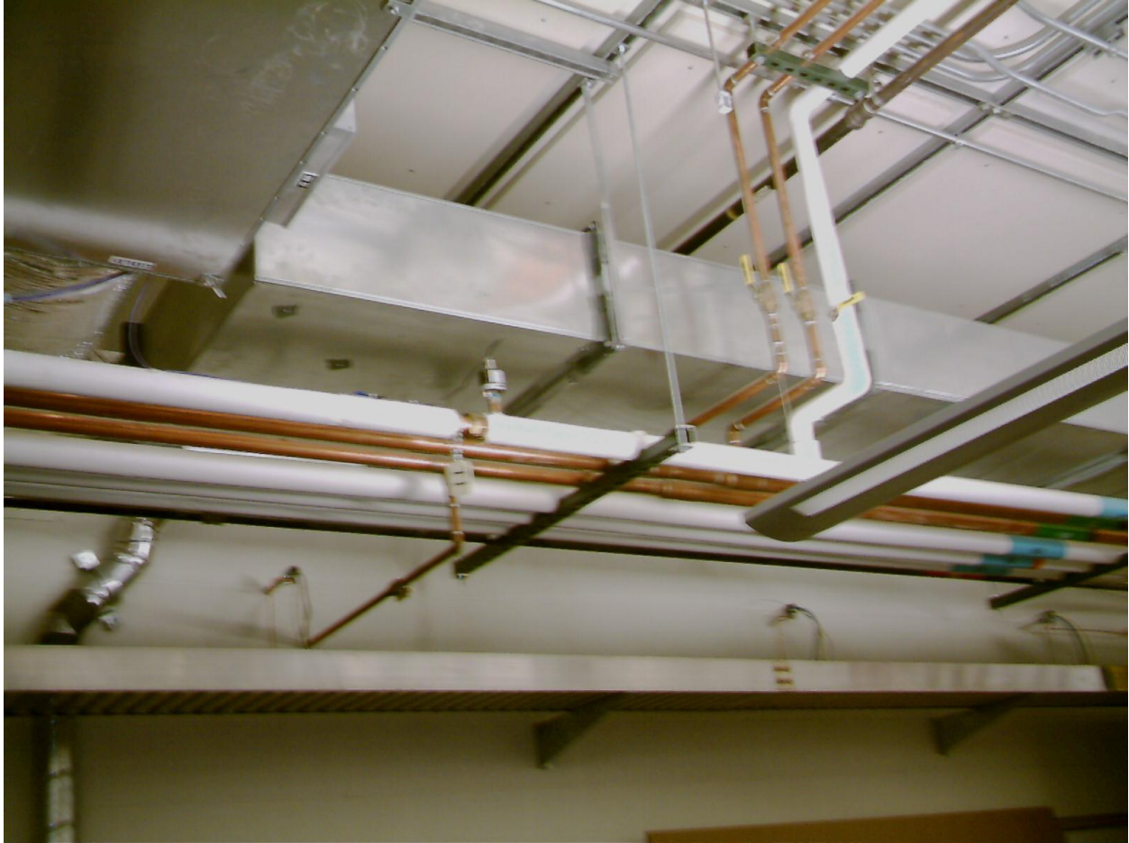
Figure 8.0, Portion of Instrumented Pipe
