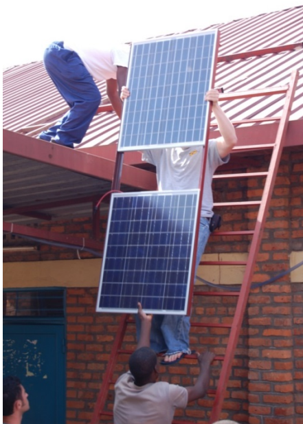
Figure 5 Unused hand railing used as a ladder.
