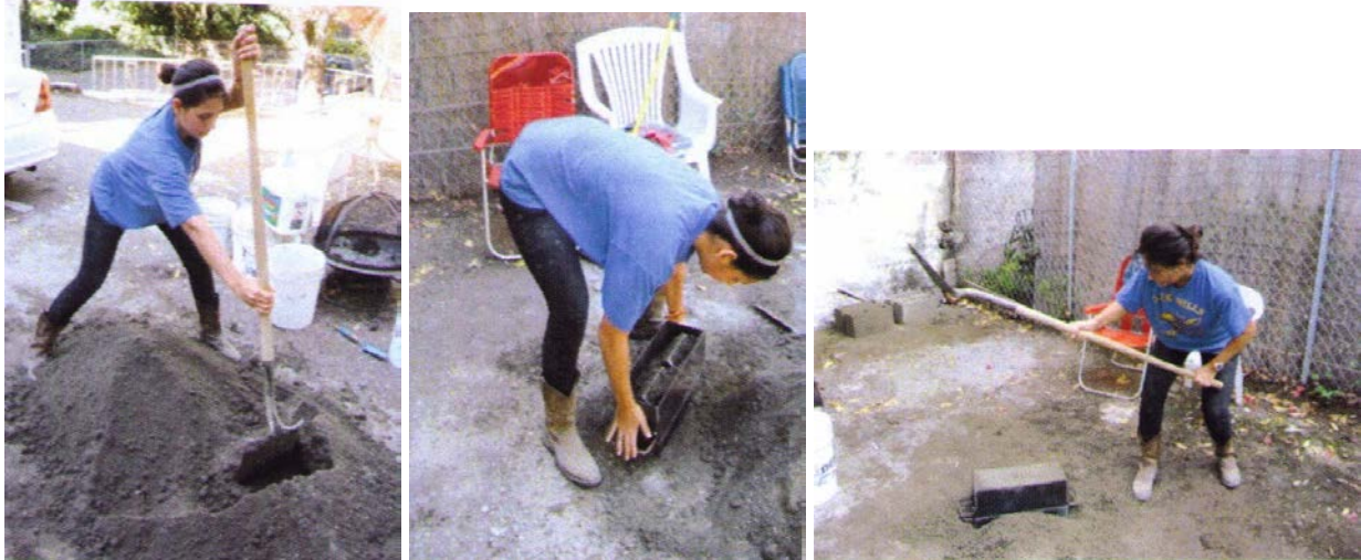
Figure 5: CMU Block Production (a) Mixing, (b) Manual Compaction and (c) Shovel Compaction
