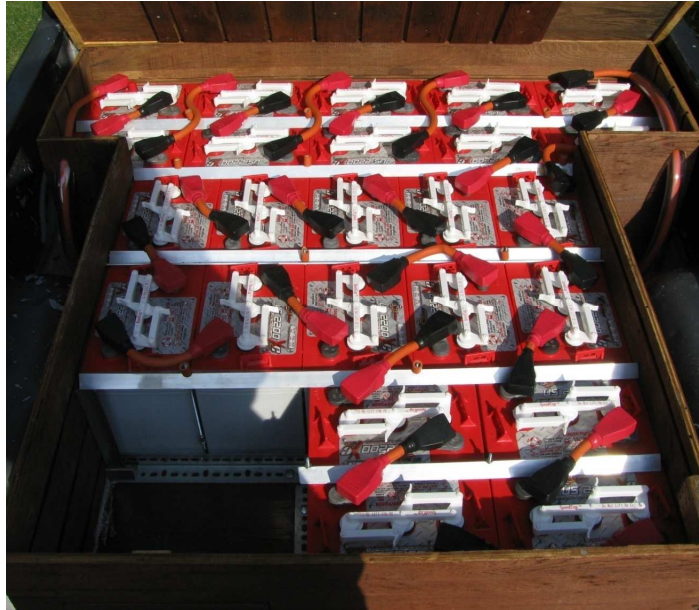
Figure 10: The Battery Compartment
