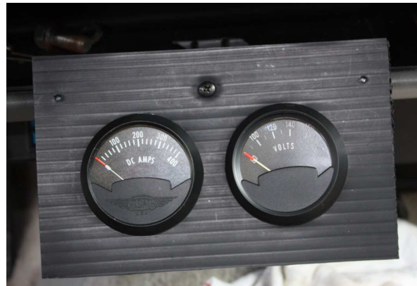
Figure 9: Voltmeter and Ammeter Gauges
