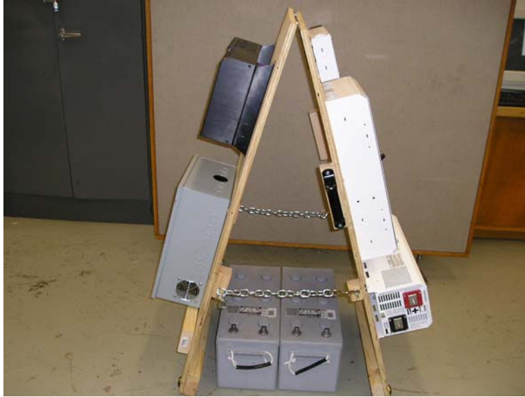
Fig. 5 Mobile module comprising a step-down transformer, C40 Charge controller, DR2424 inverter, a DC disconnect switch and a battery bank
