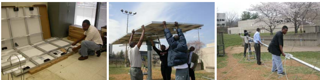
Pictures showing the students assembling and mounting the PV modules and erecting the wind turbine
