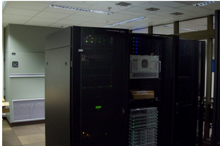
Figure 3. HPC-CRL Data Center Laboratory.
