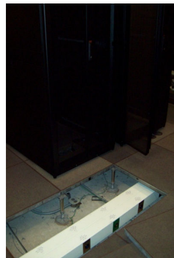
Figure 4. Data Laboratory Power Distribution.
