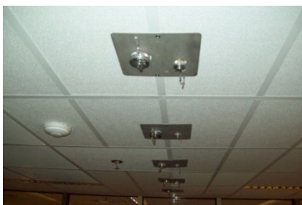
Figure 5. Data Laboratory Supplemental Cooling Manifold Ports.
