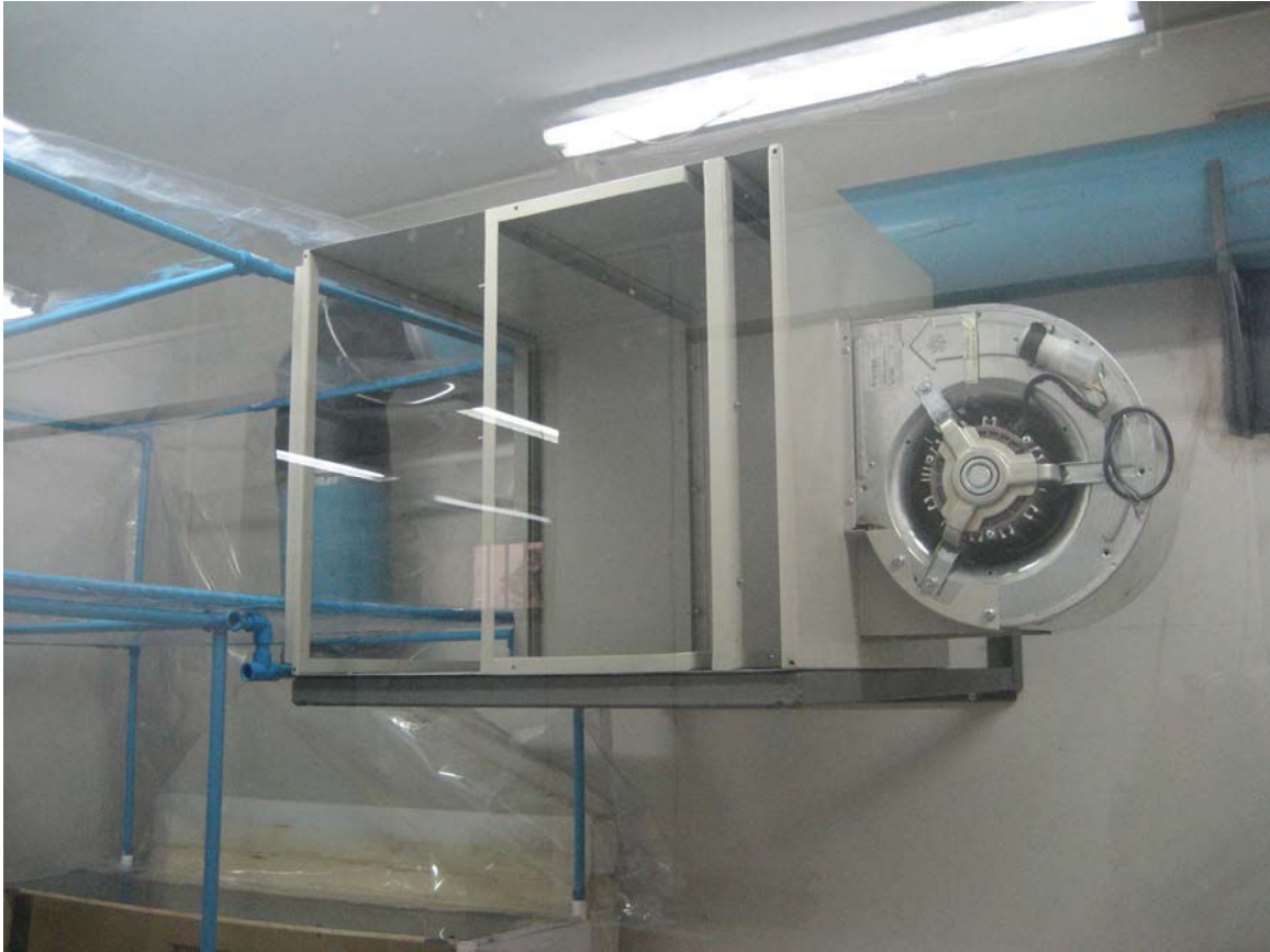
Fig. 4. The air handling unit. The filter box cover is removed, to show the slots where the prefilter, bag filter and HEPA filter are installed. Air flow into the cleanroom is from right to left. The cleanroom exhaust is visible behind the air handling unit.
