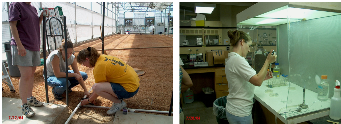
Figure 3a) Installation of the water recycle system in the hydroponics green house; b) Testing for bacteria within the system during operation.
