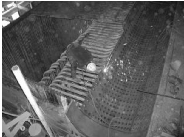
Figure 4: Inside Power Plant Boiler
