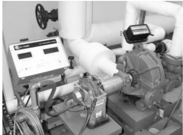
Figure 3: Carling Steam Turbine
