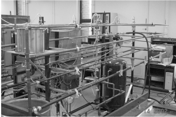
Figure 5 Pump and Piping System Experiment
