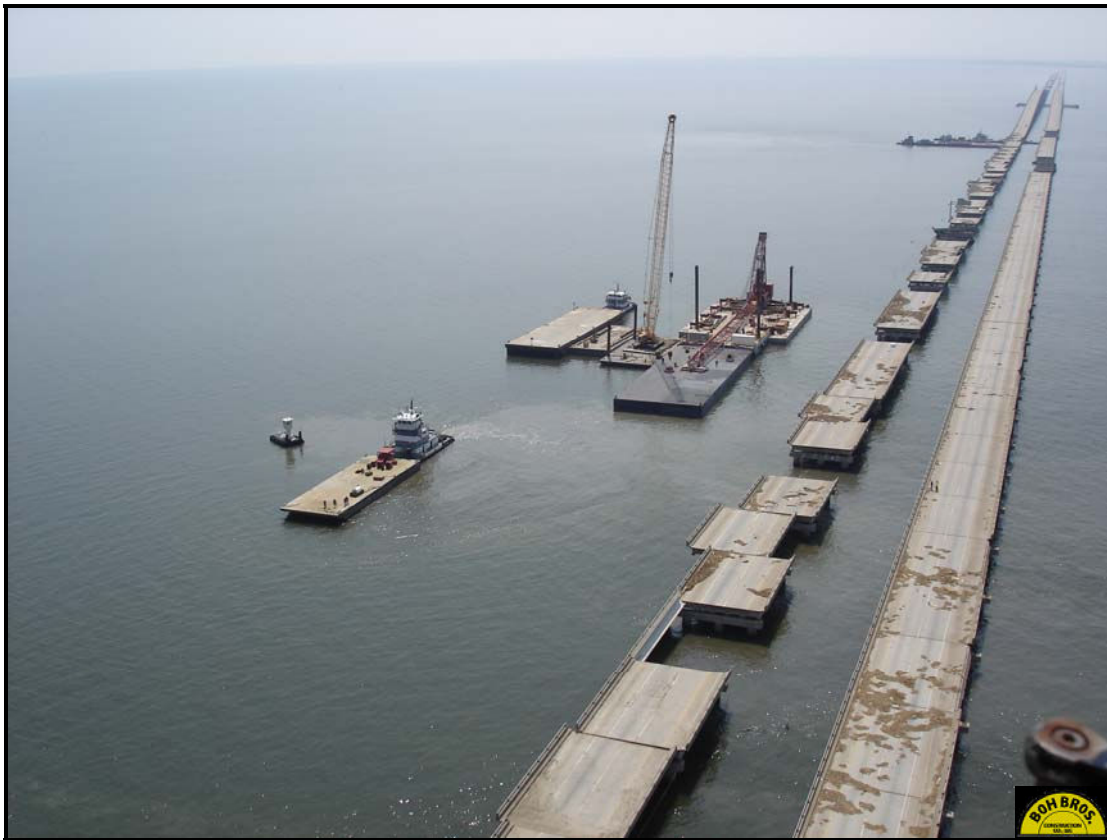
Figure 1: I-10 Bridge Damage
