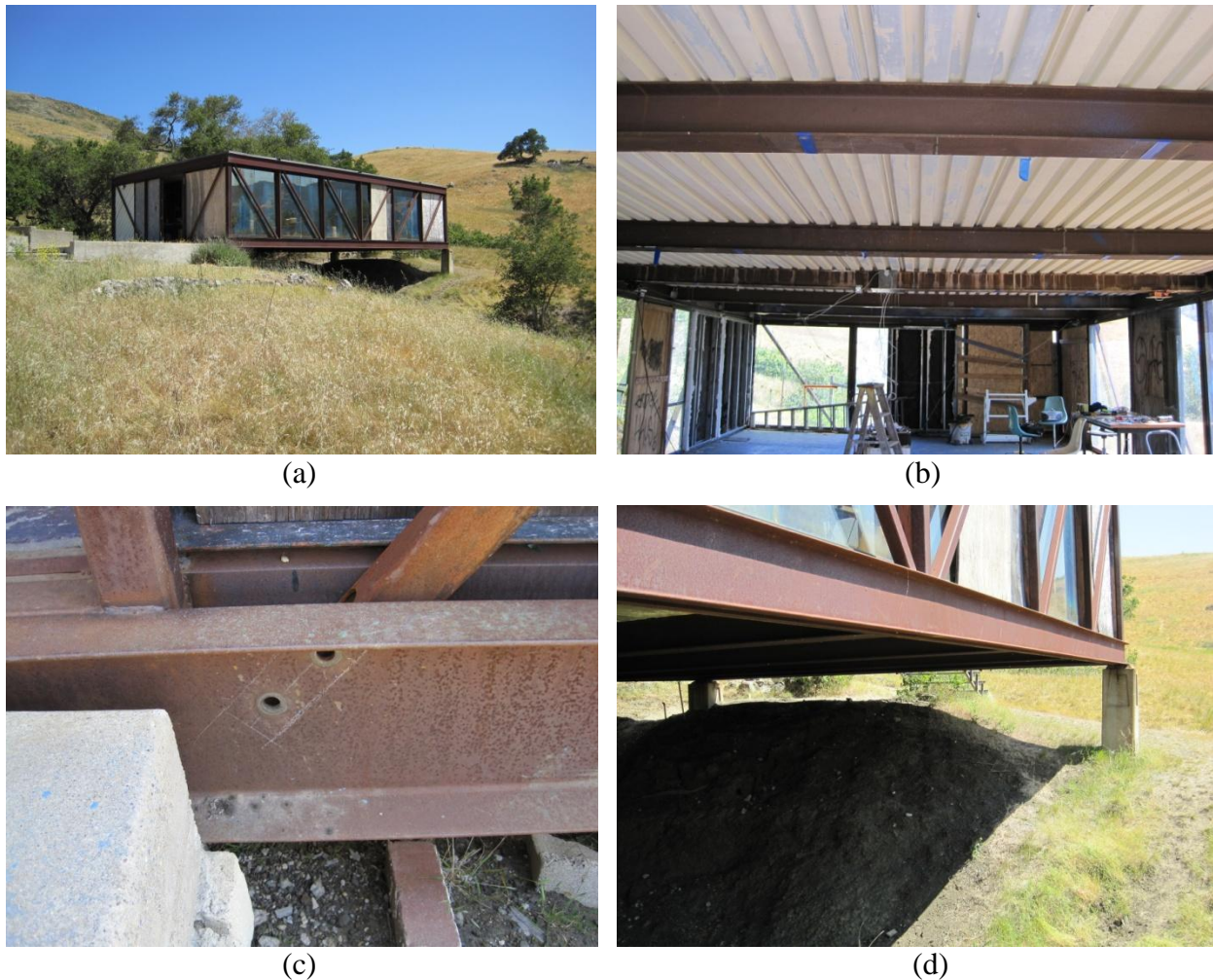
Figure 1. Bridge House (a) Exterior; (b) Interior; (c) Removable Brace Connection (N/S Direction); (d) Concrete Foundation Piers
