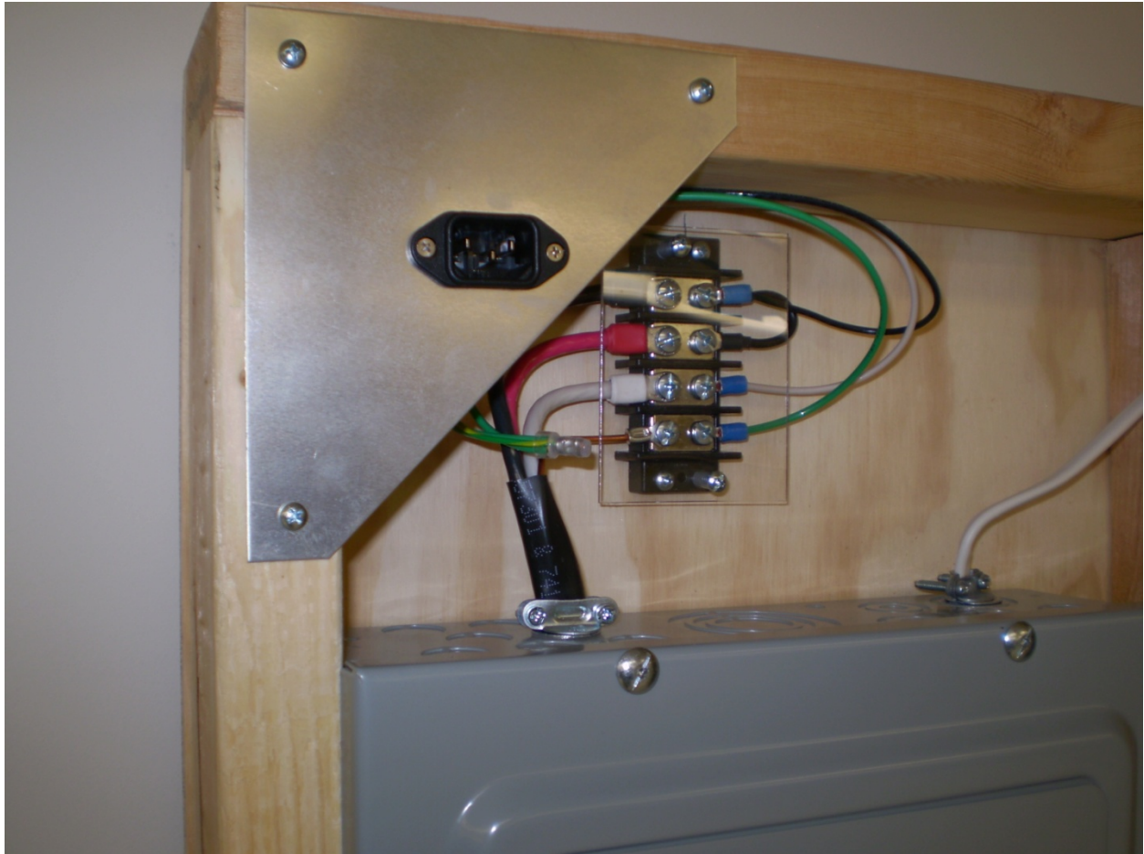
Figure 8. Electrical Power Entrance on Student Units
