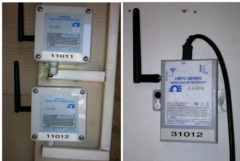
Figure 5c. Wireless transmitters and 8-Channel receiver [19-20]
