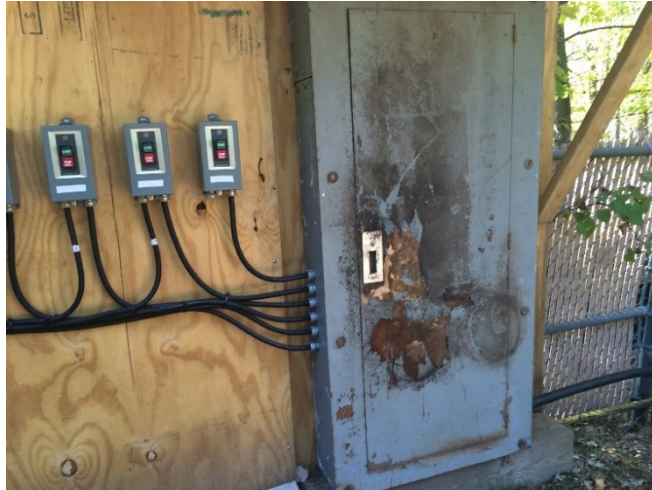
Figure 2: Original 480V Breaker Panel
