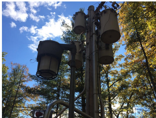
Figure 1: Original Pole-Mounted Transformers
