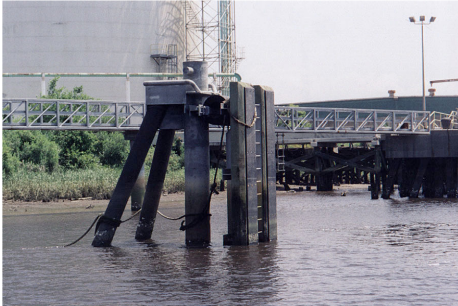
Breasting and Mooring Dolphin in Georgetown, South Carolina. This project required an energy evaluation of ship impact forces to determine the design forces, and the design of the structure to transfer 50-tons of horizontal force into soils consisting of limestone over silt.
