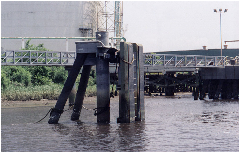
Photograph 3: Breasting and Mooring Dolphin in Georgetown, South Carolina. This project required an energy evaluation of ship impact forces to determine the design forces, and the design of the structure to transfer 50-tons of horizontal force into soils consisting of limestone over silt.
