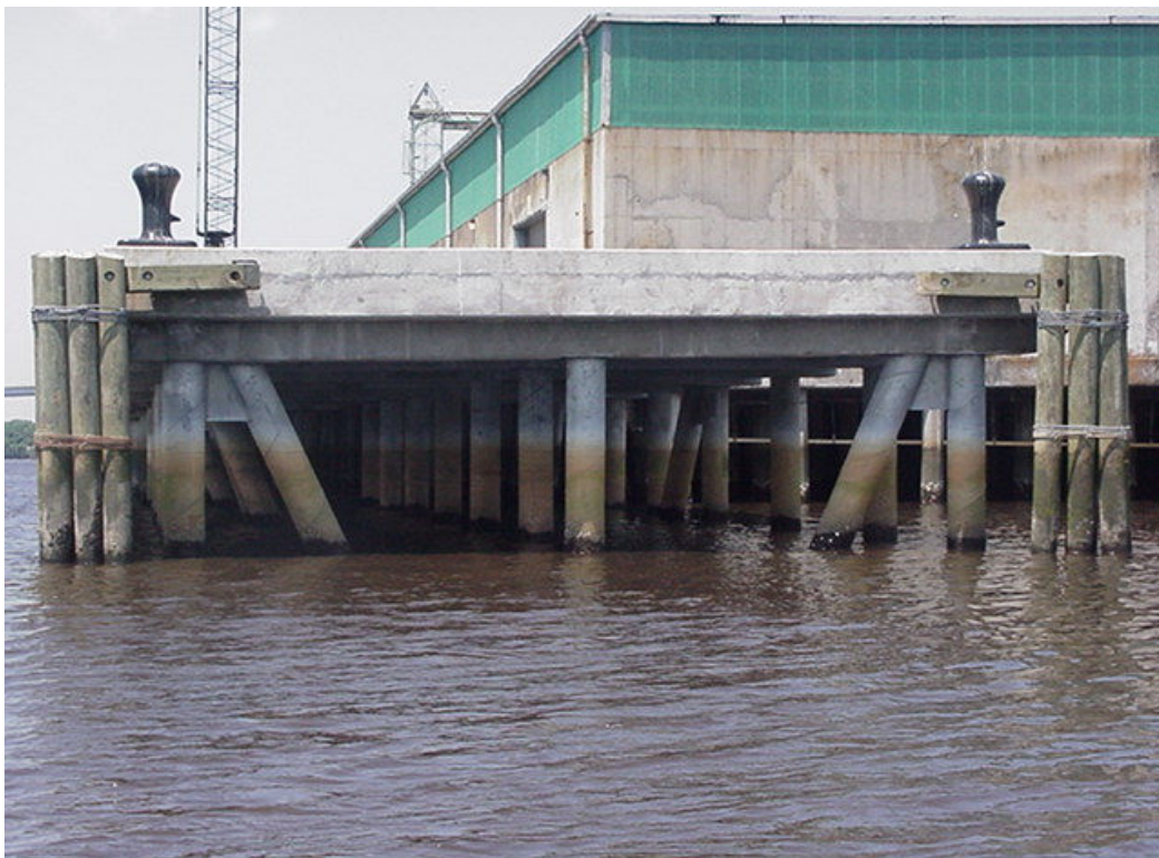
Photograph 1: Wharf Extension in Georgetown, South Carolina. This shows the vertical and batter steel pipe piles below the wharf extension.
