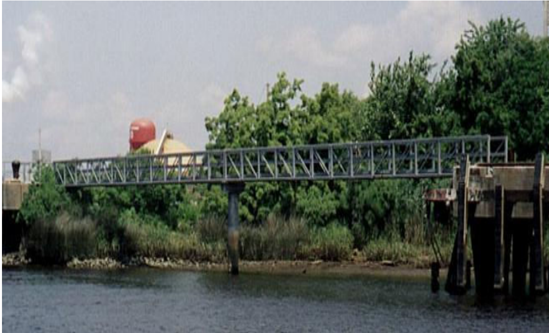
Photograph 4: Catwalk to Mooring Dolphin in Georgetown, South Carolina. This project required evaluation of a simple long span truss structure over the difficult soil conditions of shallow weak soils overlaying limestone.
