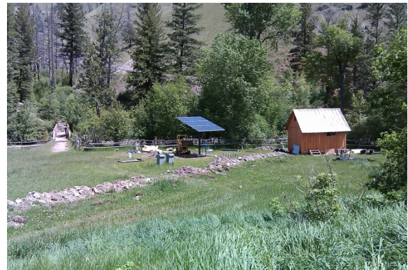
Figure 3. First solar panel installed. New power house is to the right of the solar panel.
