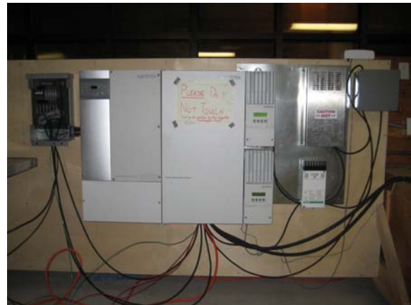
Figure 5. Central distribution, main controller, and diversion load in lab.
