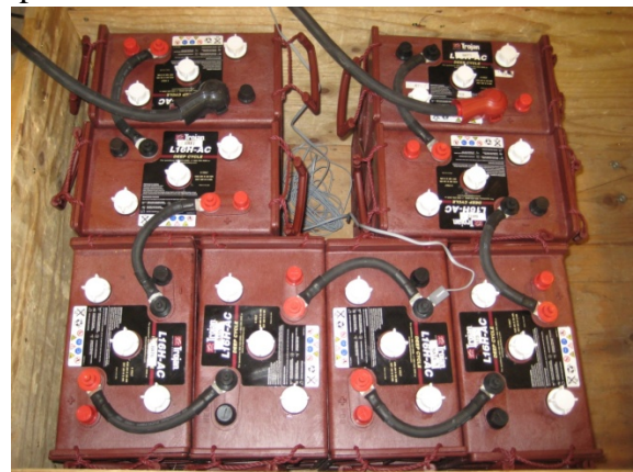
Figure 4. Battery bank in lab.
