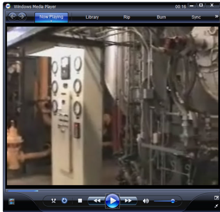
Figure 2: Portion of a walk through video of the boiler room showing the controls for one boiler.
