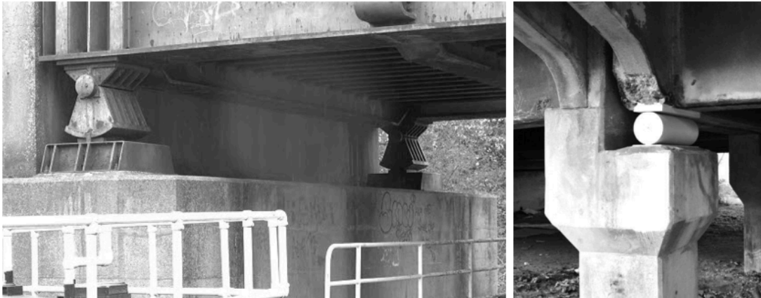
Figure 2: Two bearing bridge connections to allow for thermal expansion. The left bridge uses a rocker bearing and the right bridge is supported on a roller bearing.
