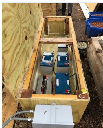
Figure 8: Battery Bank Cabinet
