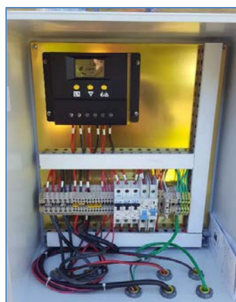
Figure 9: PV Power Panel
