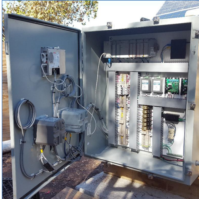
Figure 6: Aquaponics System Control Panel
