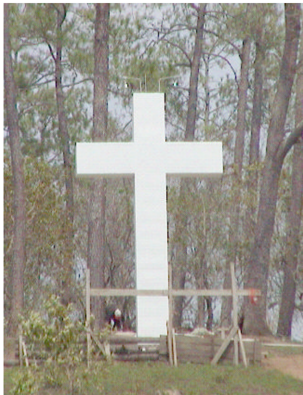
Figure 8: The cross after the formwork was stripped (top) and the final product (bottom).
