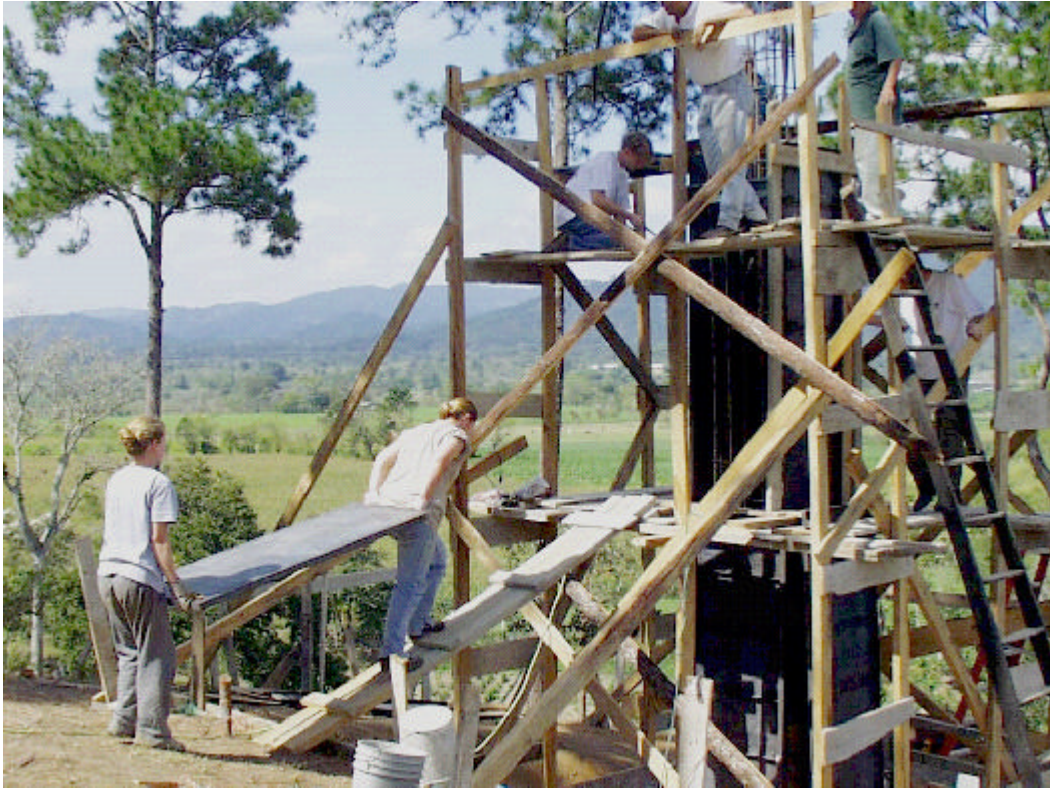
Figure 4: The second level of scaffolding is completed with a ramp to the first level.
