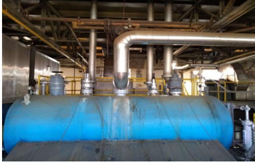
Top of Boiler, where water is pumped in
