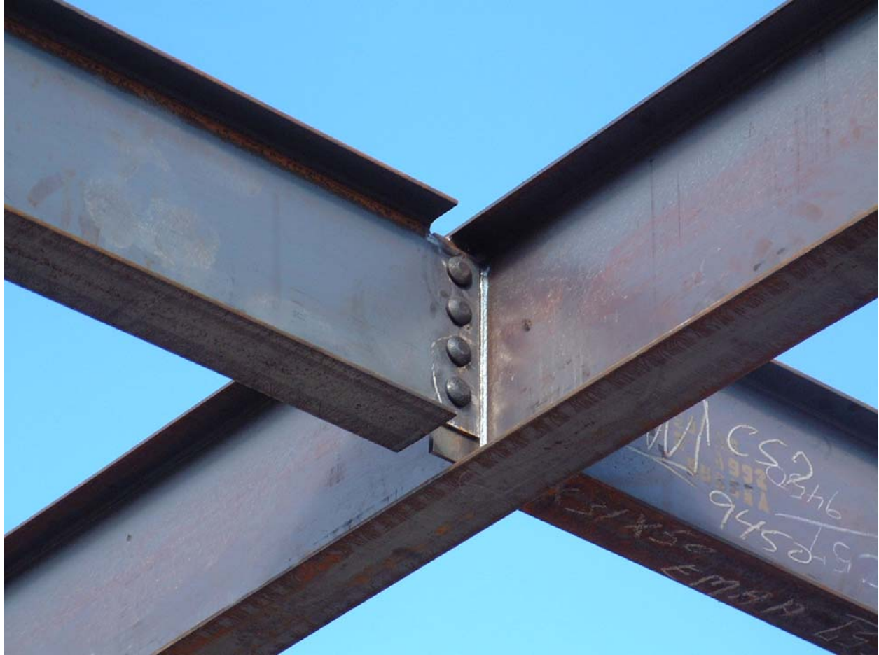
Figure 8: Two Beam Connection Using Single Plates (photograph by Edwin Schmeckpeper)
