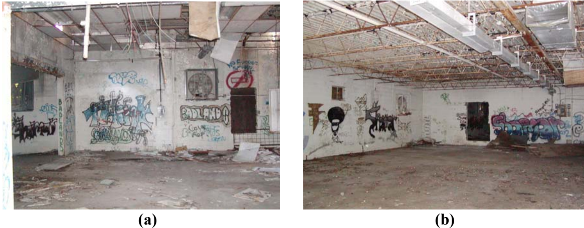
Figure 2 Graffiti on Walls, Rusted Steel Roof Trusses and Part of Collapsed Roof
