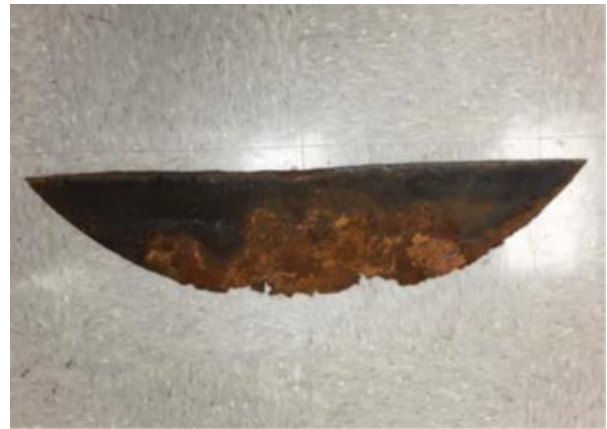
Fig. 2 Failed oil separator weir plate.
