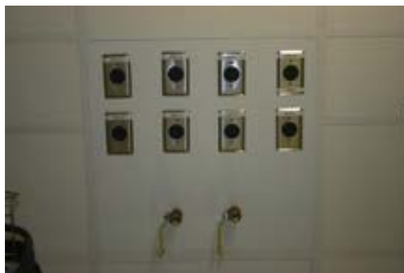
Figure 3. Utility panel supplying seven 110 V and one 208 V circuits along with compressed air and filtered water.
