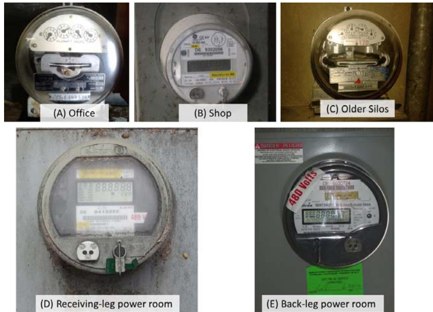
Figure 4: The five on-site power meters tracking electrical usage for billing by DTE Energy at the MAC Marlette facility. Meters (A), (B) and (C) are meters for the site office building, the work shop and the older silos used for specialty storage needs respectively. Meter (D) #9413322 tracks electric energy usage at the front area of the facility and meter (E) #6030724 tracks electronic energy usage in the back-leg receiving area of the facility. These two latter meters track the bulk of the energy usage at the Marlette facility. These meters provide power service to the areas indicated in Figure 5 below.
