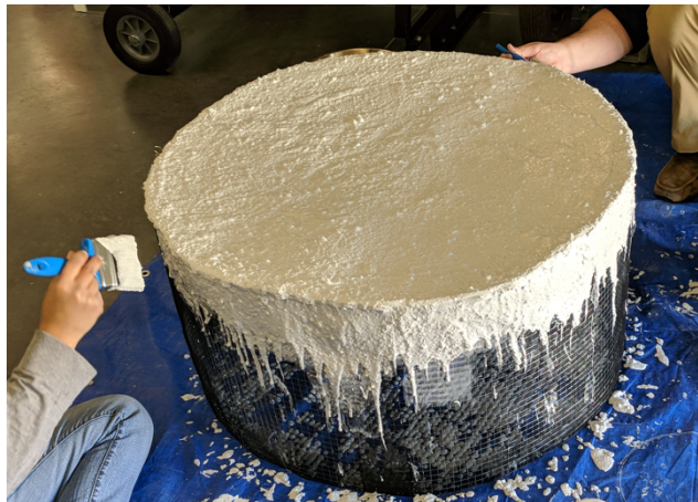
Figure 1- Building the acrylic concrete rainwater harvesting tank at the construction workshop phase of the project.
